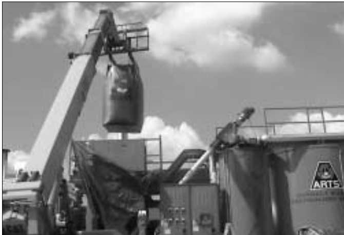
Rubber is poured into the hopper and blended with the liquid asphalt.
